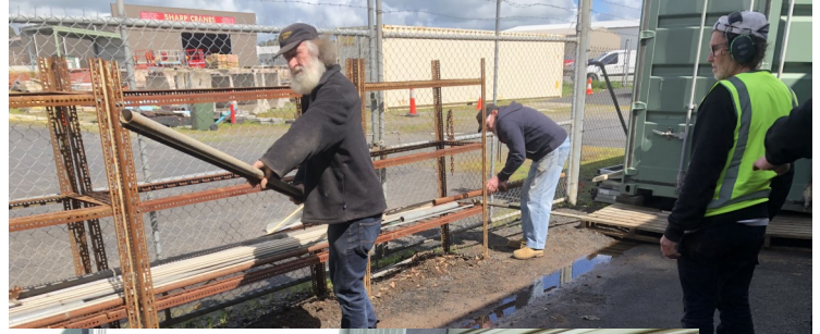
Removing steel storage rack in readiness for canopy over containers for outdoor workspace
