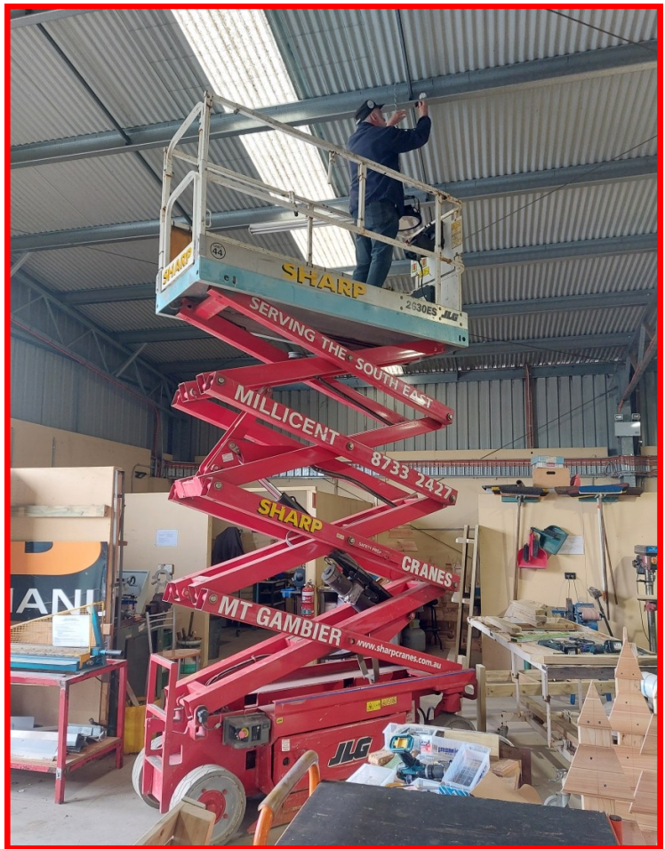
Rob B, our qualified electrician, replacing an LED light Thanks to our sponsor for the machine
